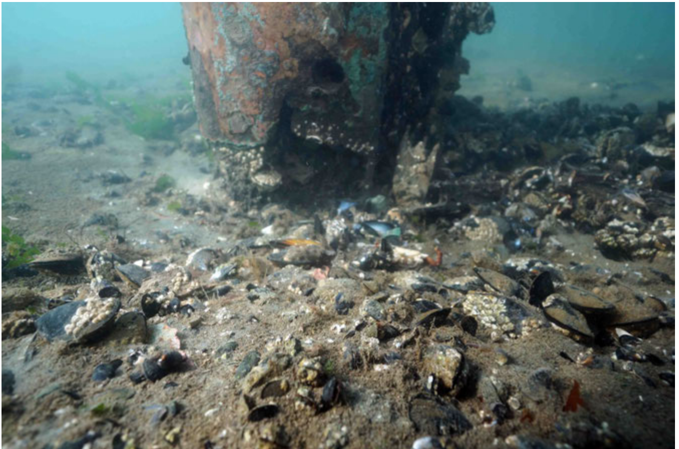
Pile 15C: Poor Condition – 50% loss of section within tidal zone
