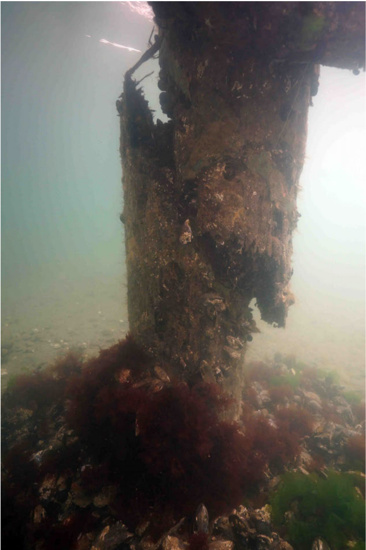
Pile 28C: Very Poor Condition – broken pile
