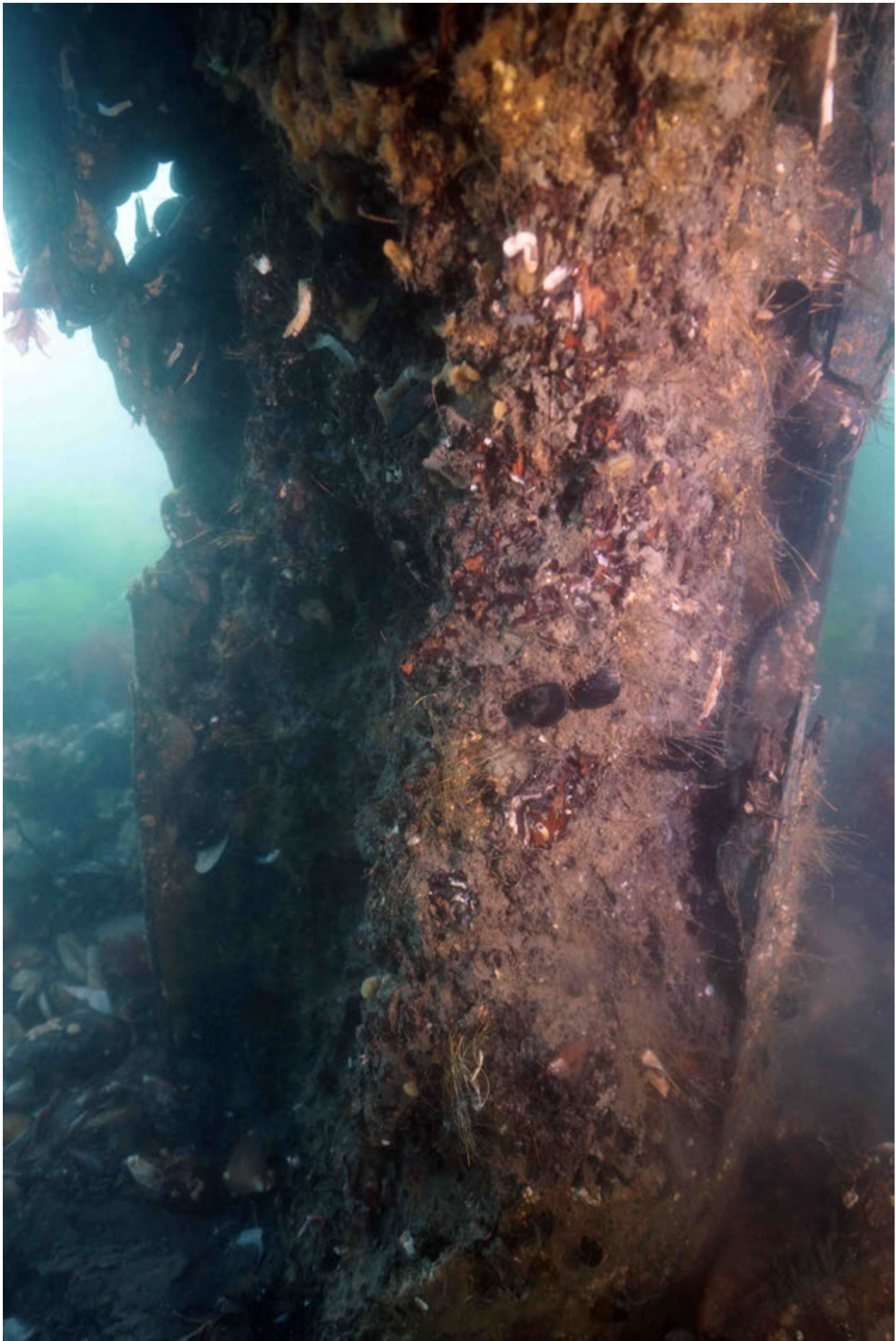
Pile 31D: Poor Condition – 60% loss of section – at seabed
