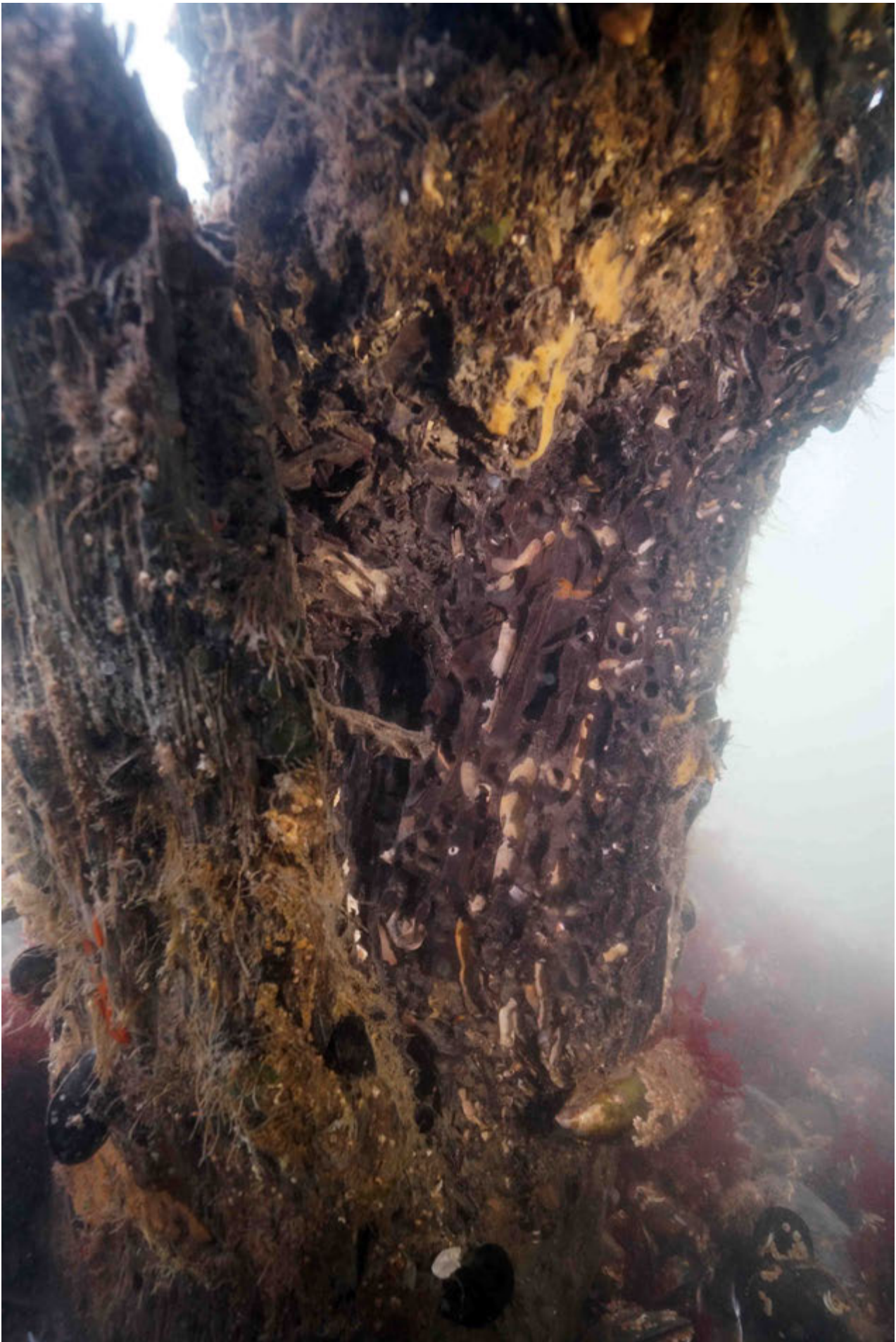
Pile 27C: Very Poor Condition – broken pile
