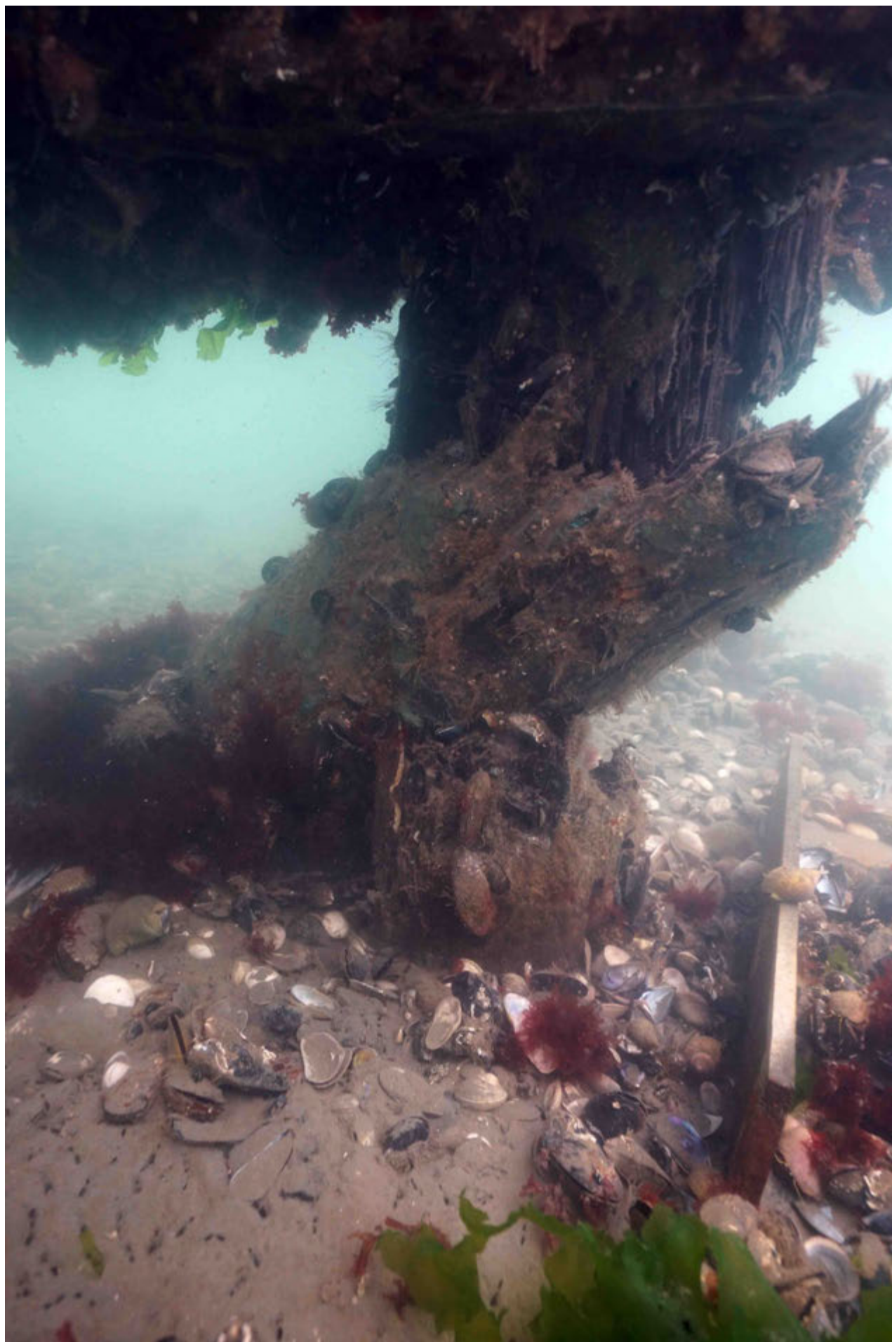
Pile 29C: Very Poor Condition – broken pile
