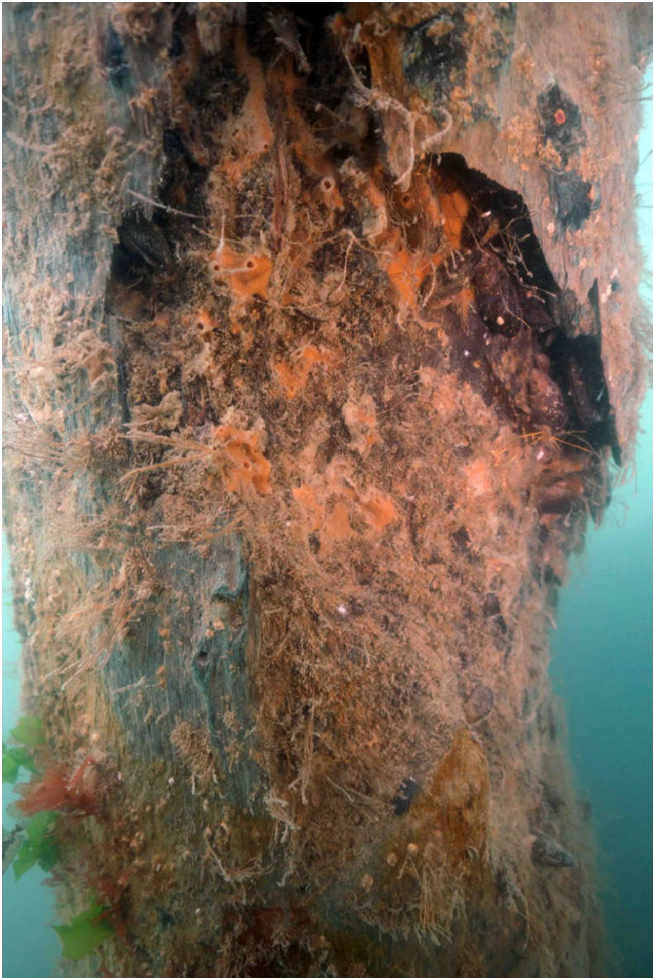
Pile 35C: Poor Condition – 40% loss of section – lower tidal zone
