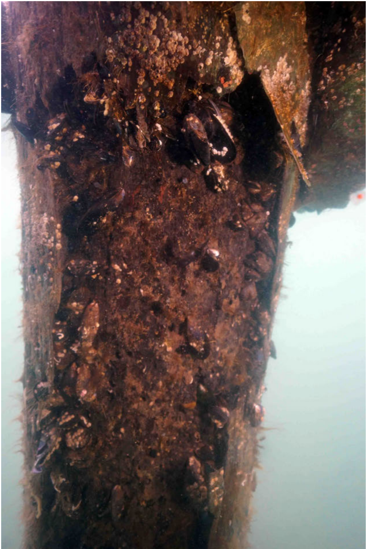
Pile 30C: Poor Condition – 40% loss of section – lower tidal zone
