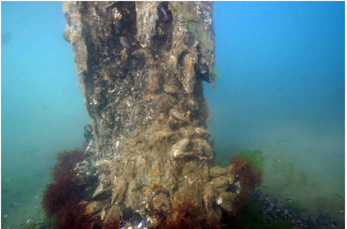
Pile 22D: Poor Condition – 60% loss of section at seabed
