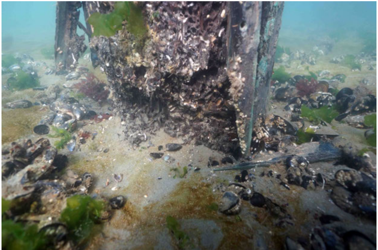
Pile 18C: Poor Condition – 50% loss of section within tidal zone
