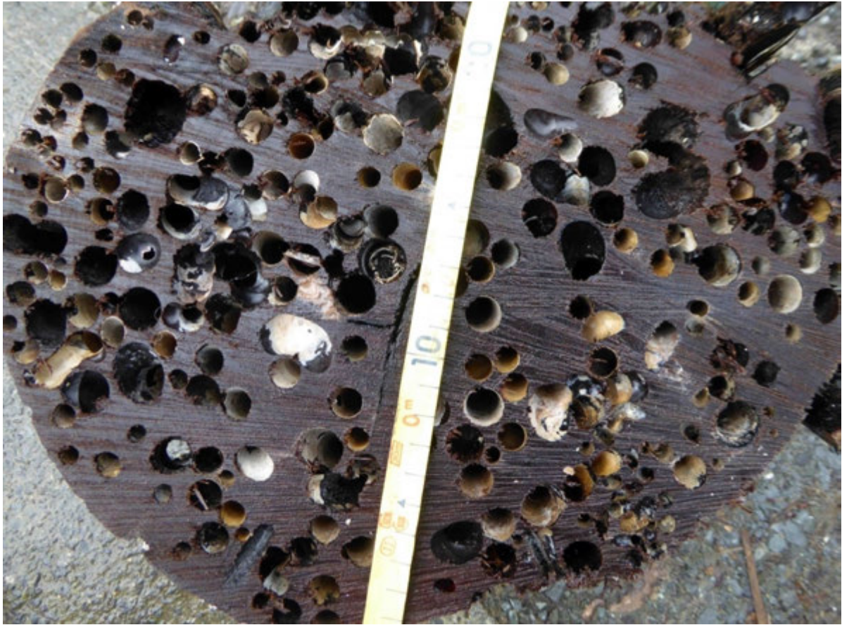
Example (from Petone Wharf) of how the Molluscan Borer 'Teredo' damages the hardwood timber piles internal integrity by significantly reducing the piles strength and mass
