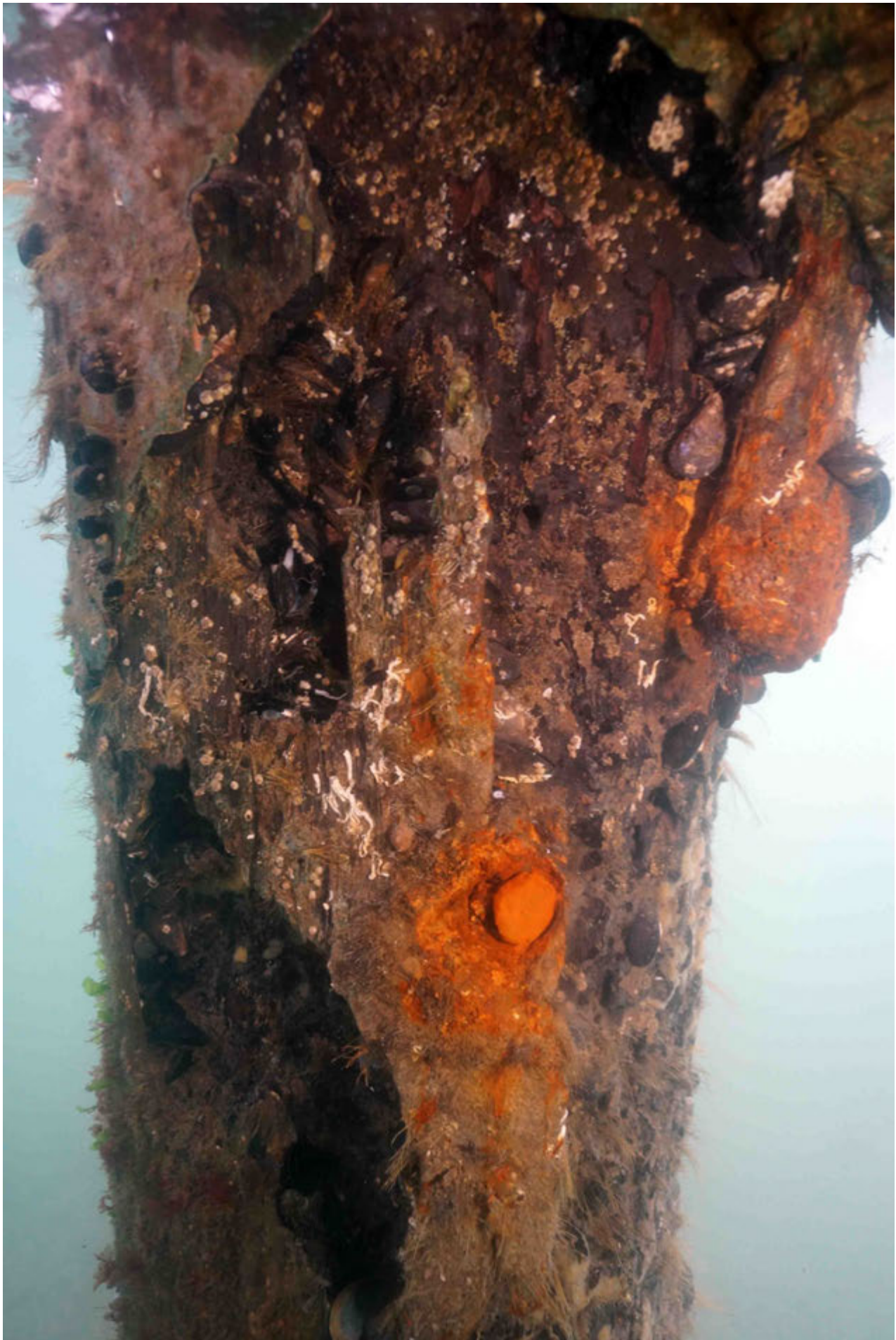
Pile 30D: Poor Condition – 50% loss of section – lower tidal zone
