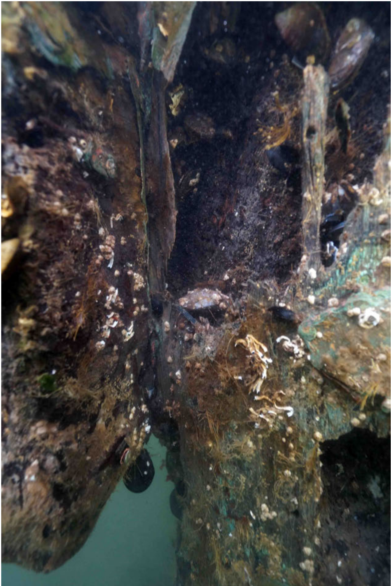
Pile 26F: Poor Condition – 60% loss of section – lower tidal zone
