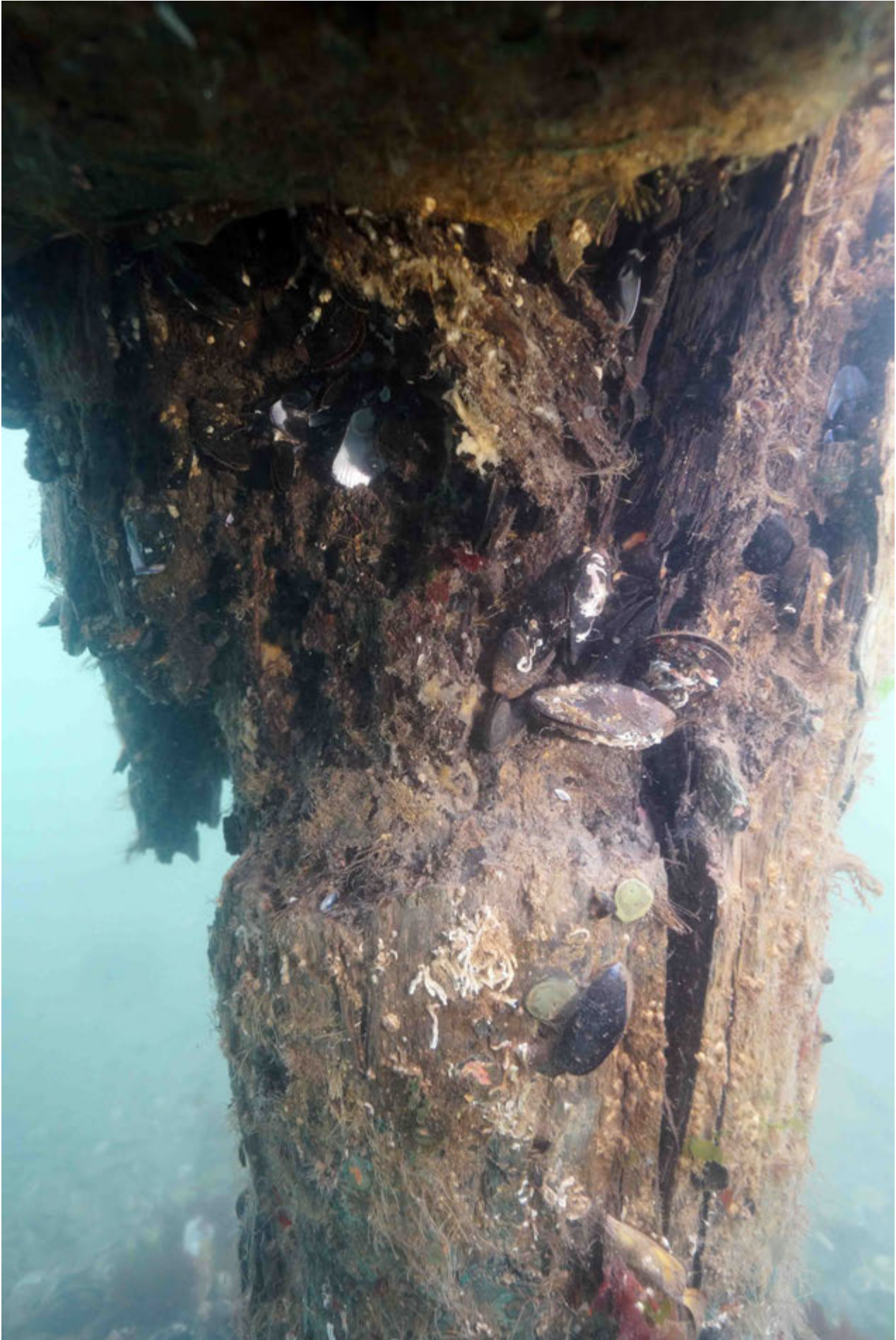
Pile 28D: Very Poor Condition – broken pile
