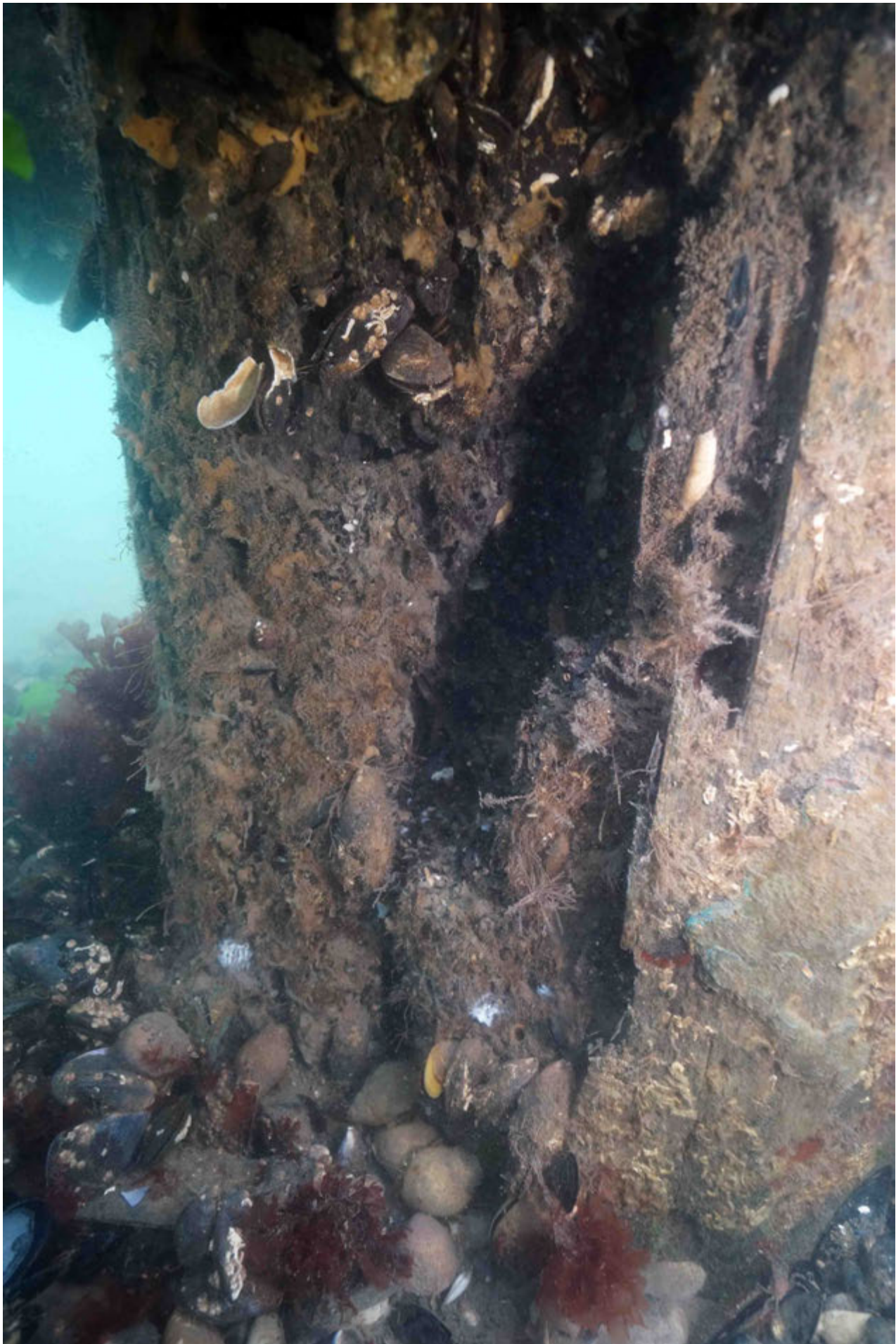
Pile 29D: Very Poor Condition – broken pile
