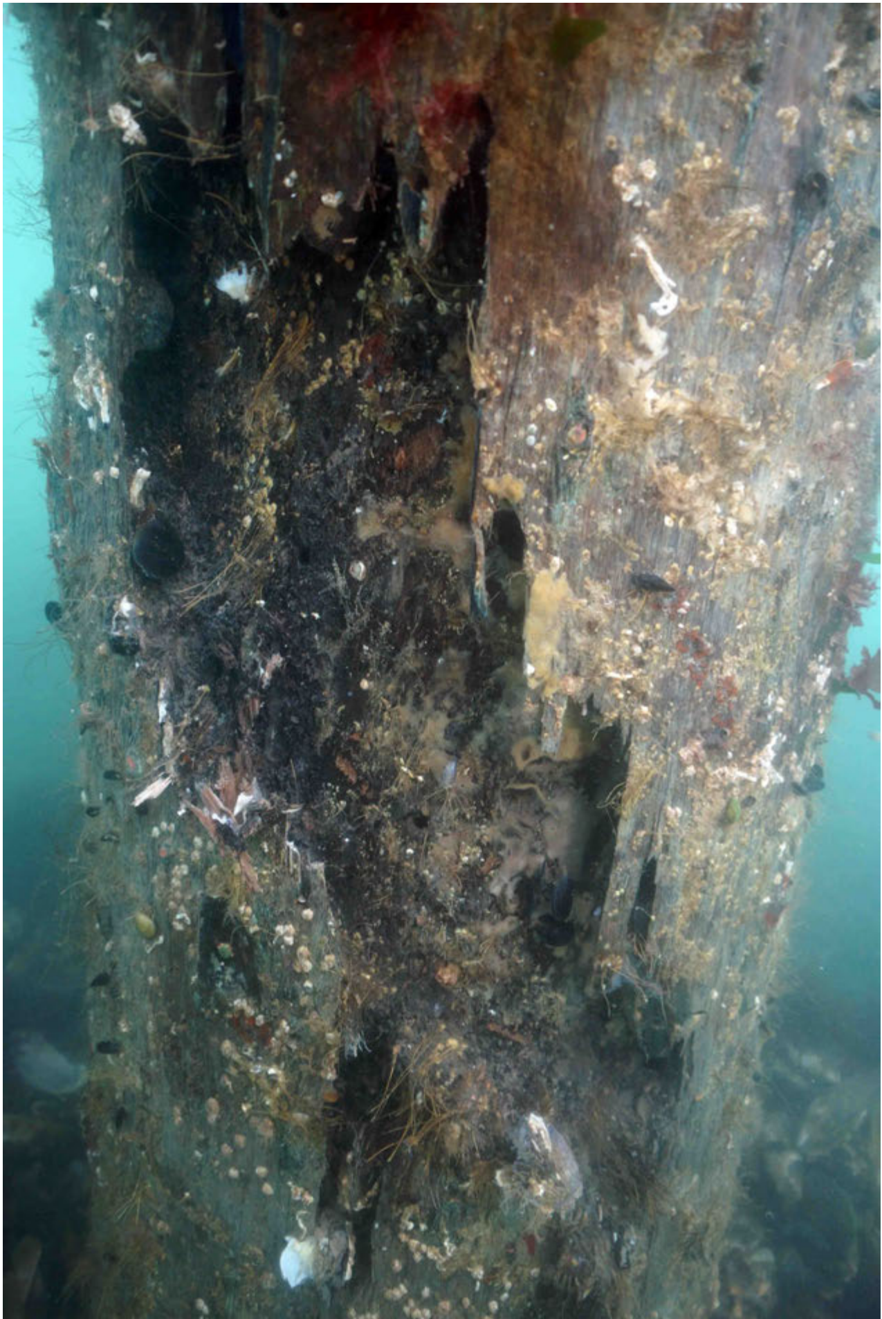
Pile 31C: Poor Condition – 40% loss of section – lower tidal zone to seabed
