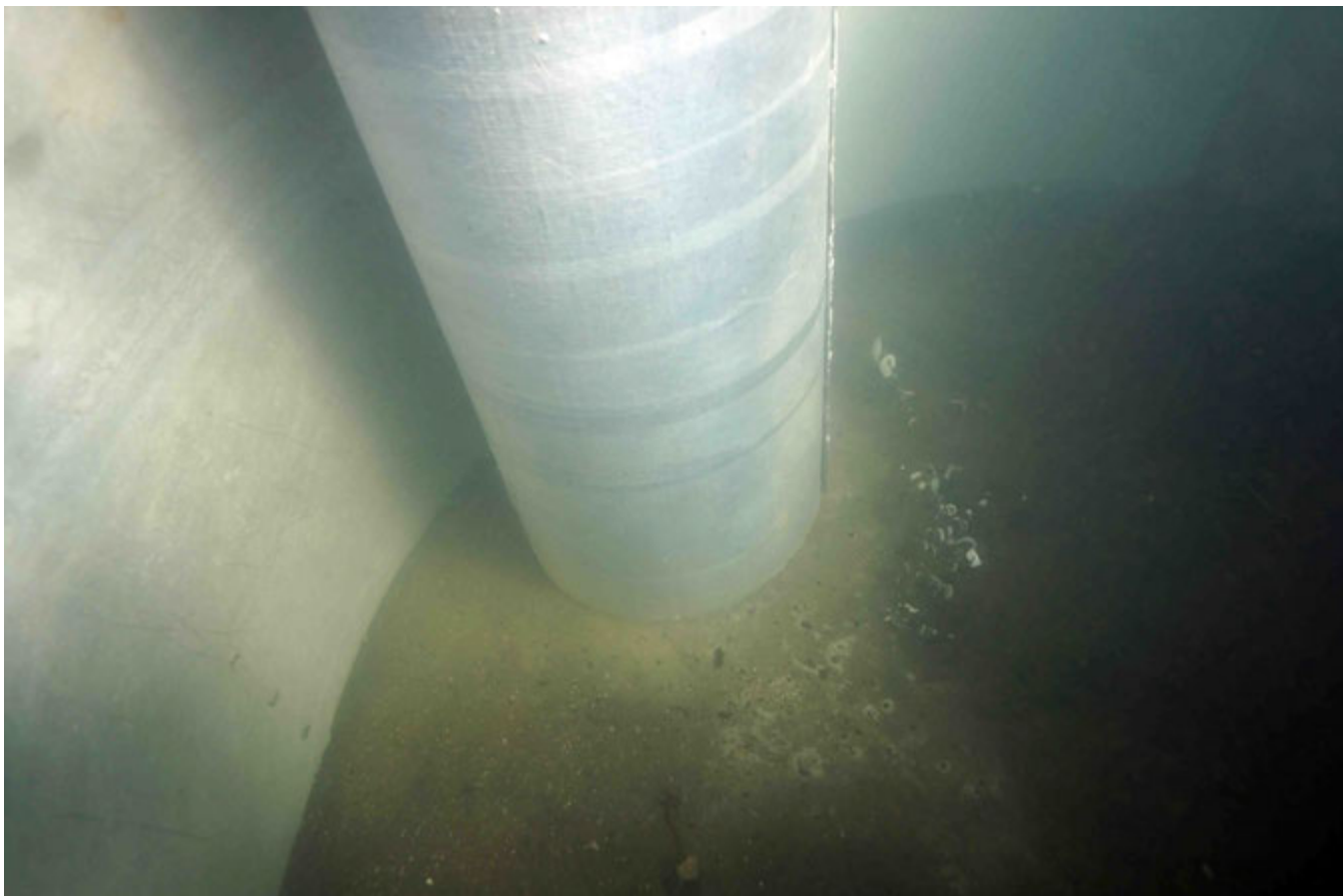
Pile 16C: Very Poor Condition – broken pile – FRP stump repair completed 13/01/2021
