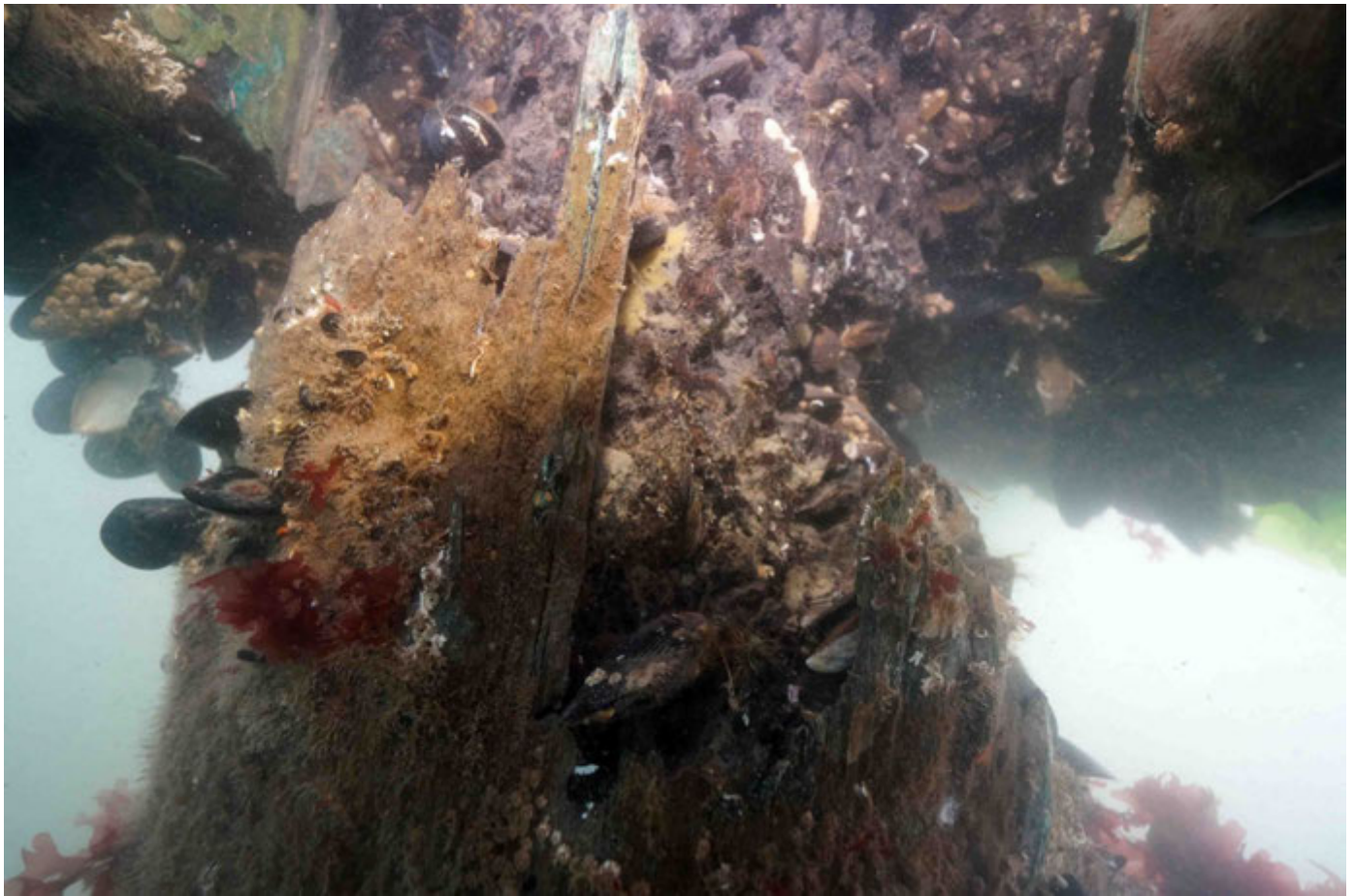
Pile 25D: Poor Condition – 60% loss of section within tidal zone
