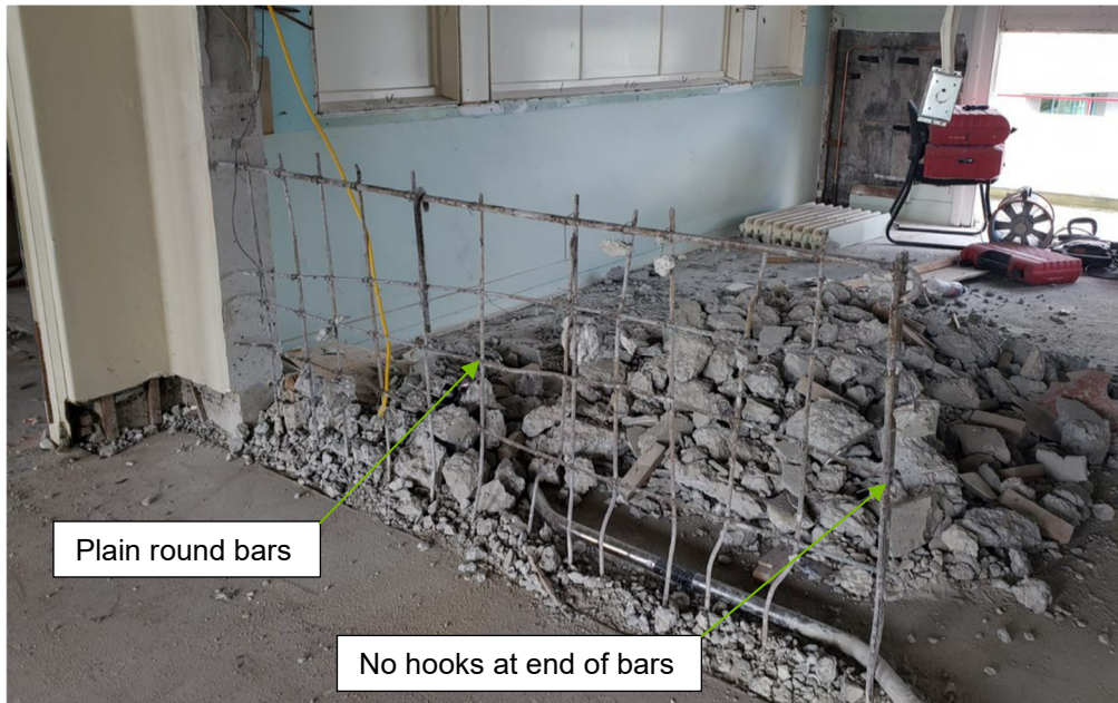
Figure 1-4 Demolished wall example showing plain round bars with no hooks at the ends of the wall
